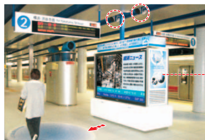
The super-directional speakers (indicated by red circles) for high-frequency sound reproduction are installed on the ceiling of the platform. Sound from these speakers can be heard only by people standing in a limited area designated by a floor sheet (indicated by the arrow). [Screen image is simulated.]
