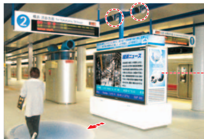
The super-directional speakers (indicated by red circles) for high-frequency sound reproduction are installed on the ceiling of the platform. Sound from these speakers can be heard only by people standing in a limited area designated by a floor sheet (indicated by the arrow). [Screen image is simulated.]
